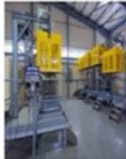
Gas Bottling Unit
