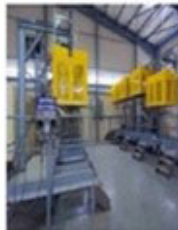
Gas Bottling Unit
