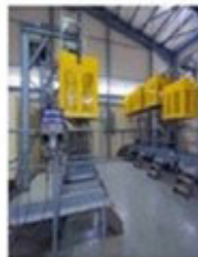
Gas Bottling Unit
